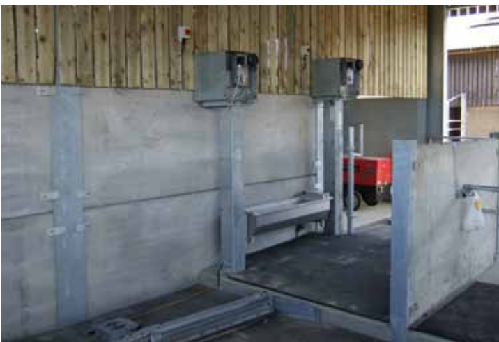
• 2 drive units, mounted on console, inside the building
