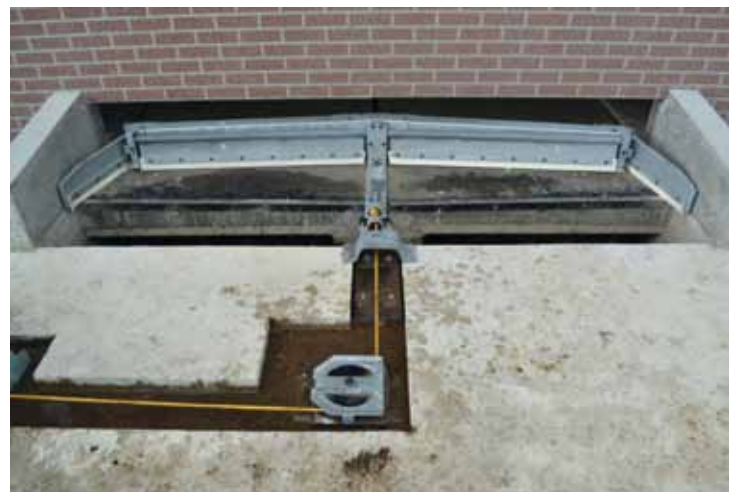
• Dump unit, located outside the building
